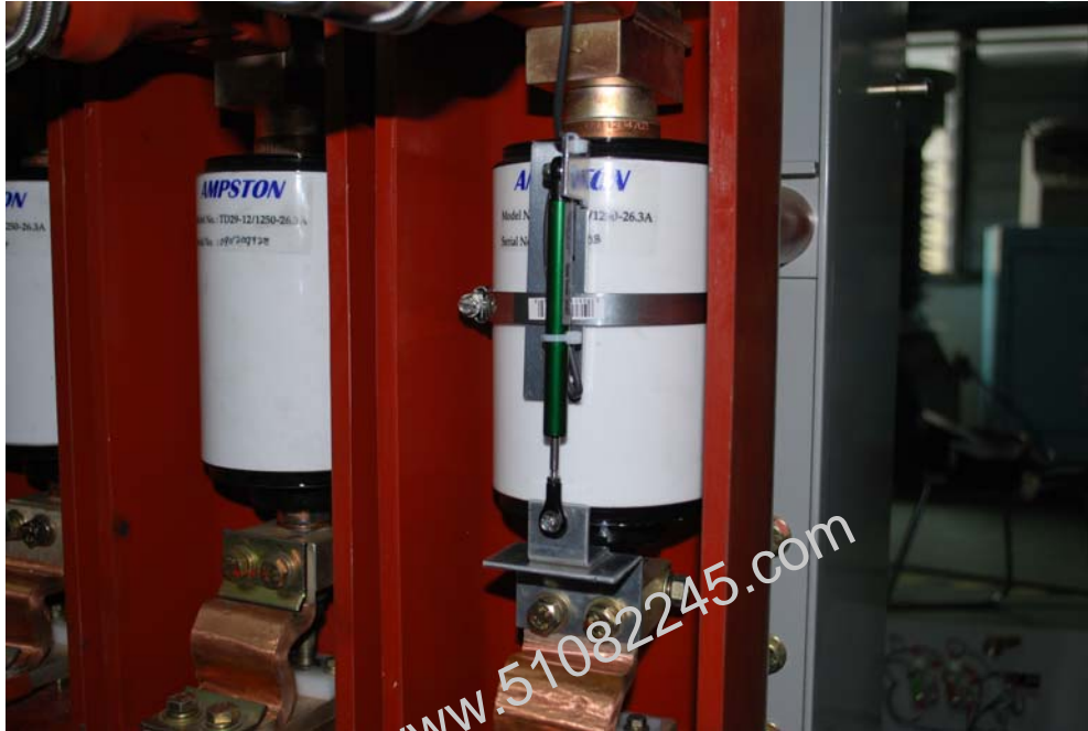
Resistor Transducer on Vacuum Circuit Breaker
