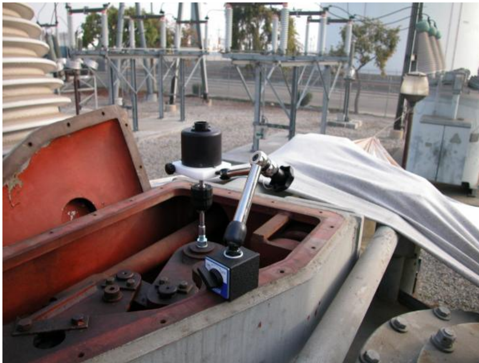
Rotary Transducer on Federal Pacific Circuit Breaker
