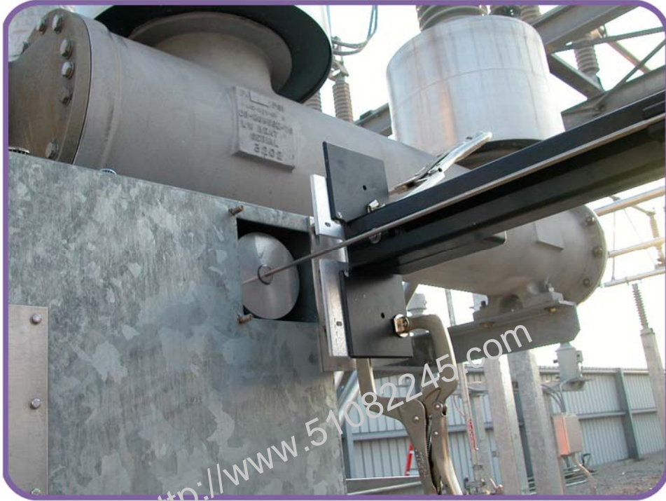
Figure 34. Linear Transducer on Areva DT1-72.5F
