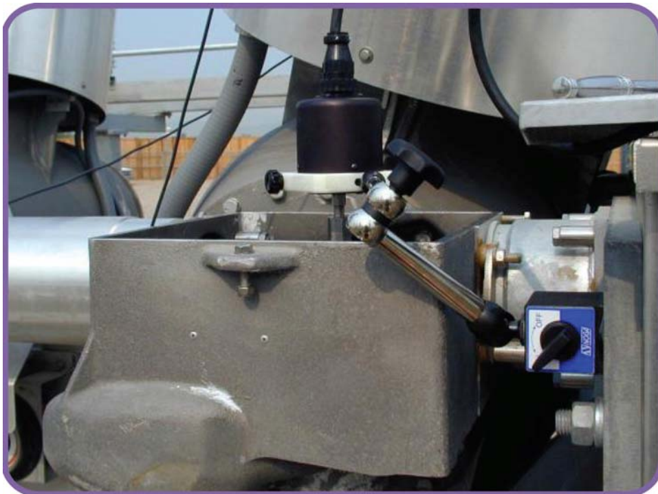
Figure 27. Rotary Transducer on Alstom HE 1014 Circuit Breaker
