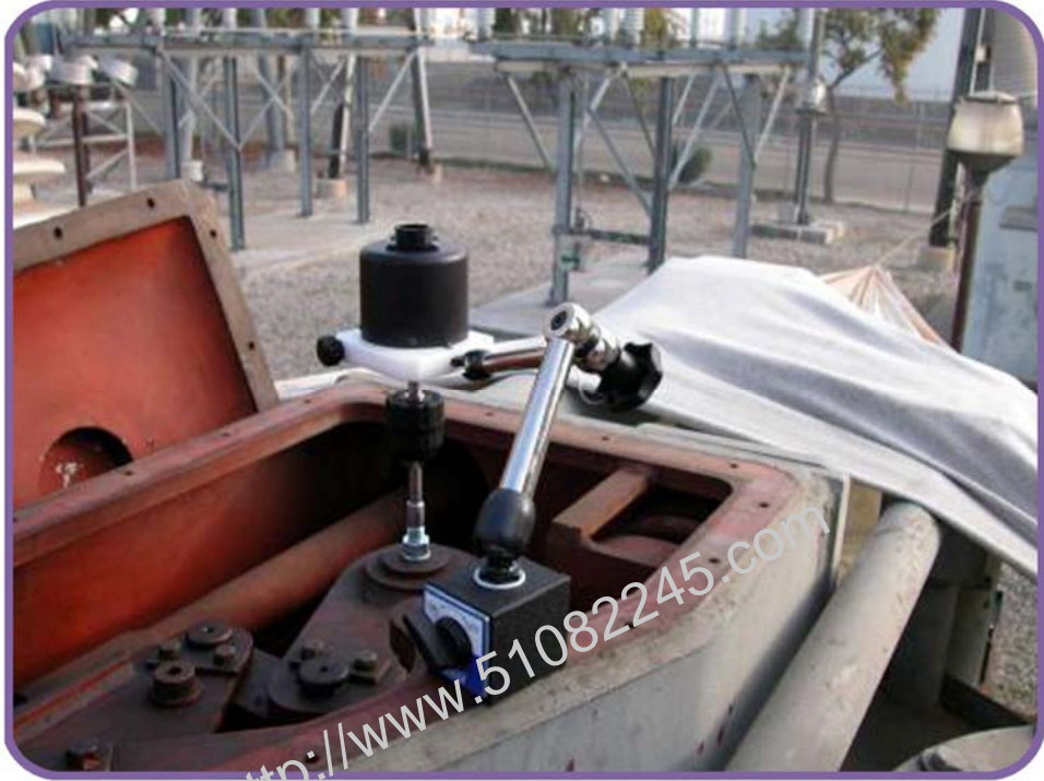
Figure 32. Rotary Transducer on Federal Pacific Breaker
