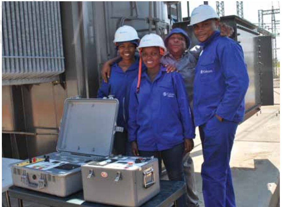
EZCT S2A and Tri-Phase at Eskom, South Africa
